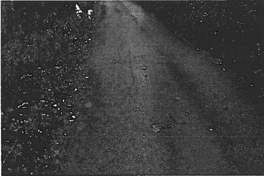
9. Depression and cracking of access road pavement along top of slope.
