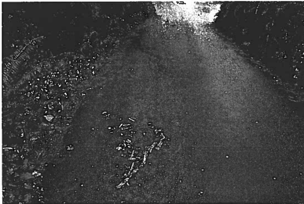
10. Depression and cracking of access road pavement along top of slope.
