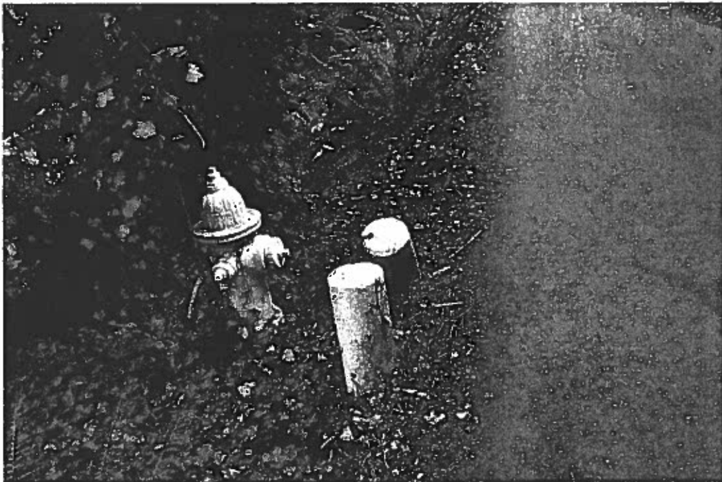
8. Leaning fire hydrant along shared access road.
